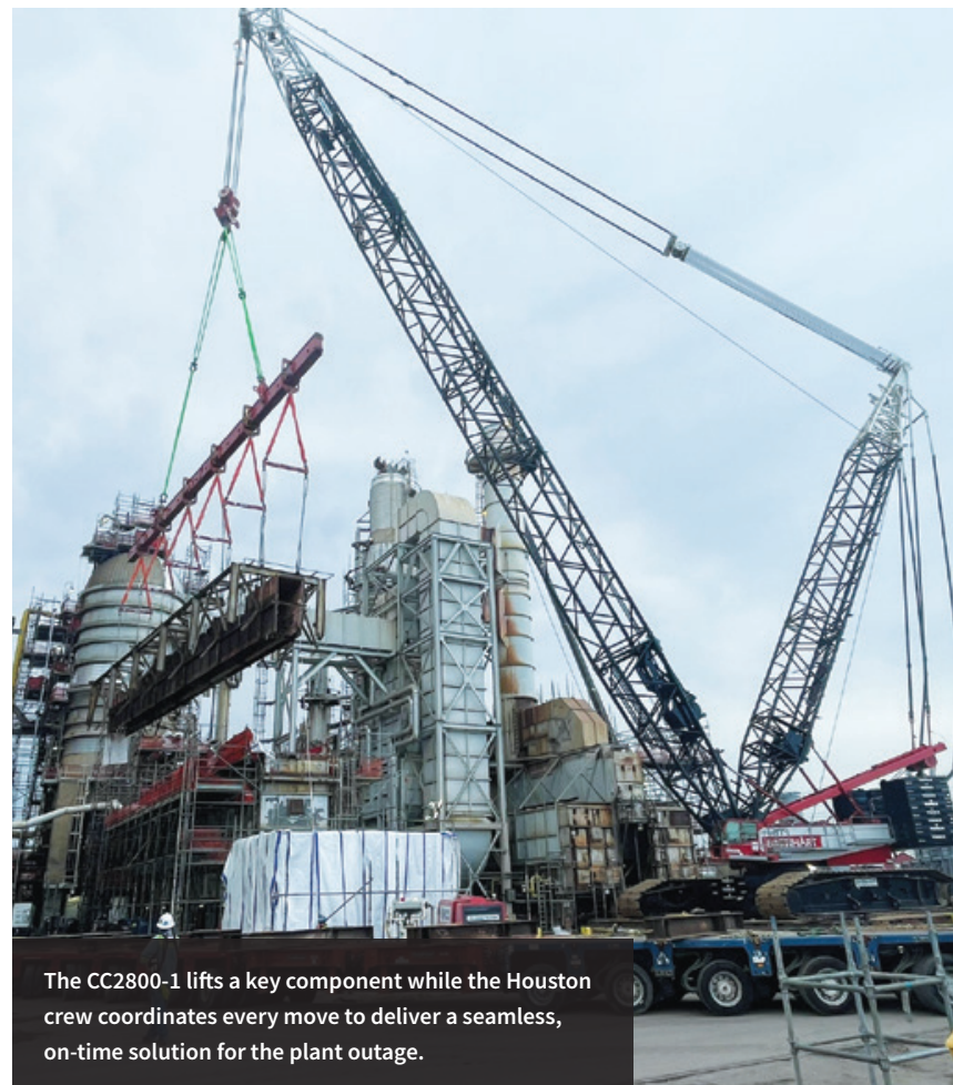
The heavy-lift CC2800-1 moves a massive plant component during a critical turnaround, working in sync with six other cranes to keep the outage on schedule.
