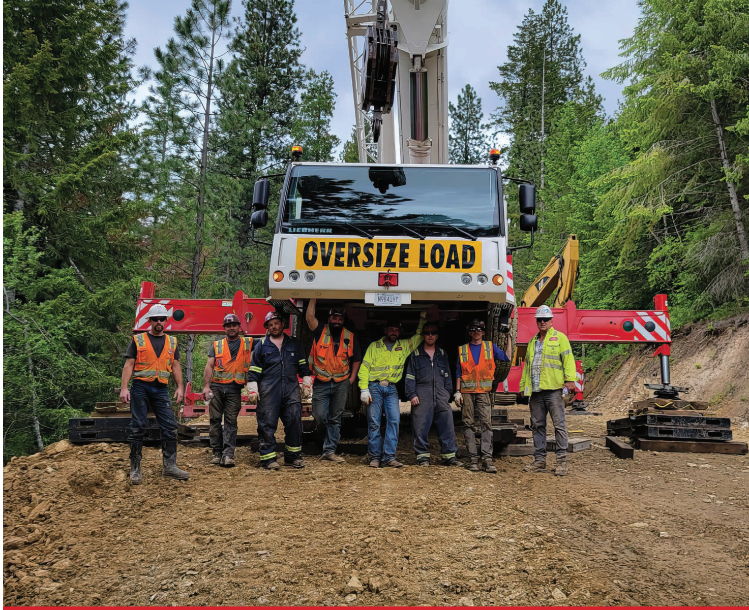
Spokane's team in the North Idaho National Forest on a project to recover a concrete mixing truck that rolled off the mountain road. The team utilized its 265-ton all-terrain Liebherr crane to turn over and hoist the fully loaded concrete truck out of the woods.
