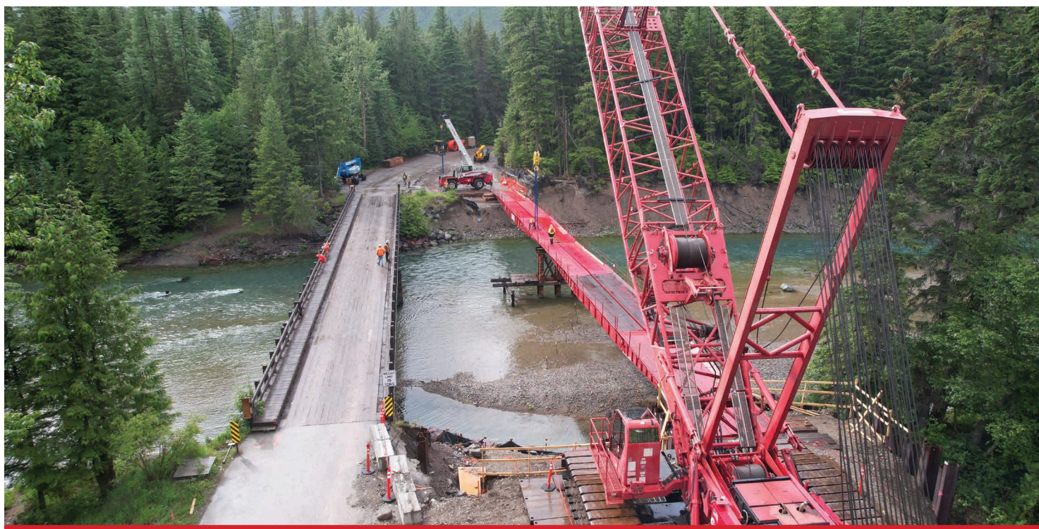
The Spokane crew helps construct a temporary bridge outside Glacier National Park (see project profile on page 9).
