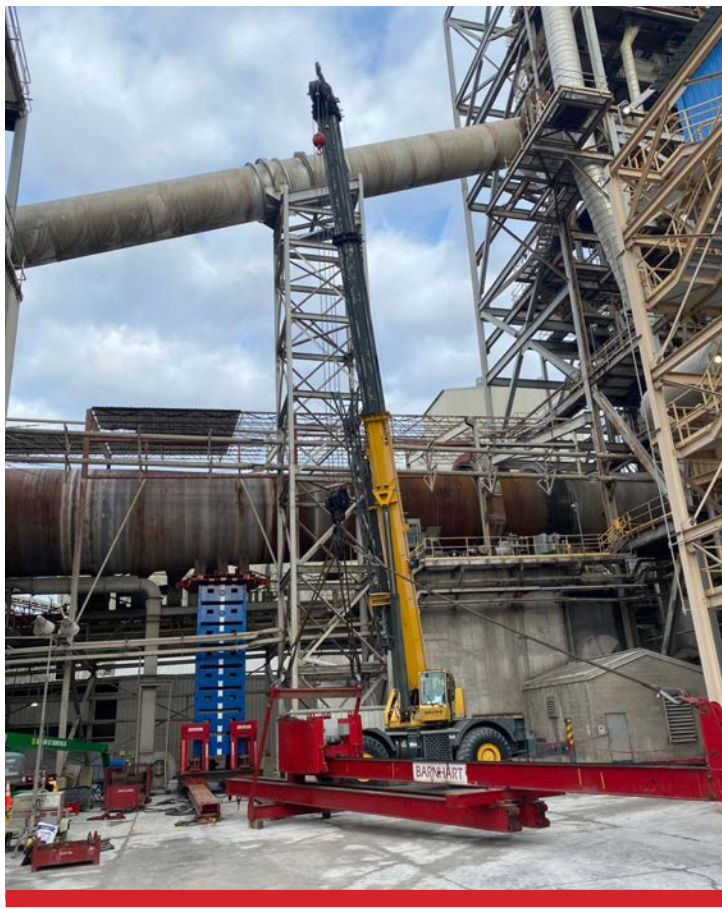
The shoring tower was slid beneath the kiln, gradually taking on the load, until it was supported properly.
