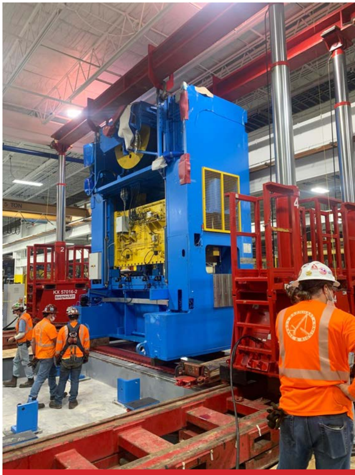
4 The press was moved on a slide system over to the pit and set into place. There were mere inches of clearance between the press and the header beams and roof steel.
