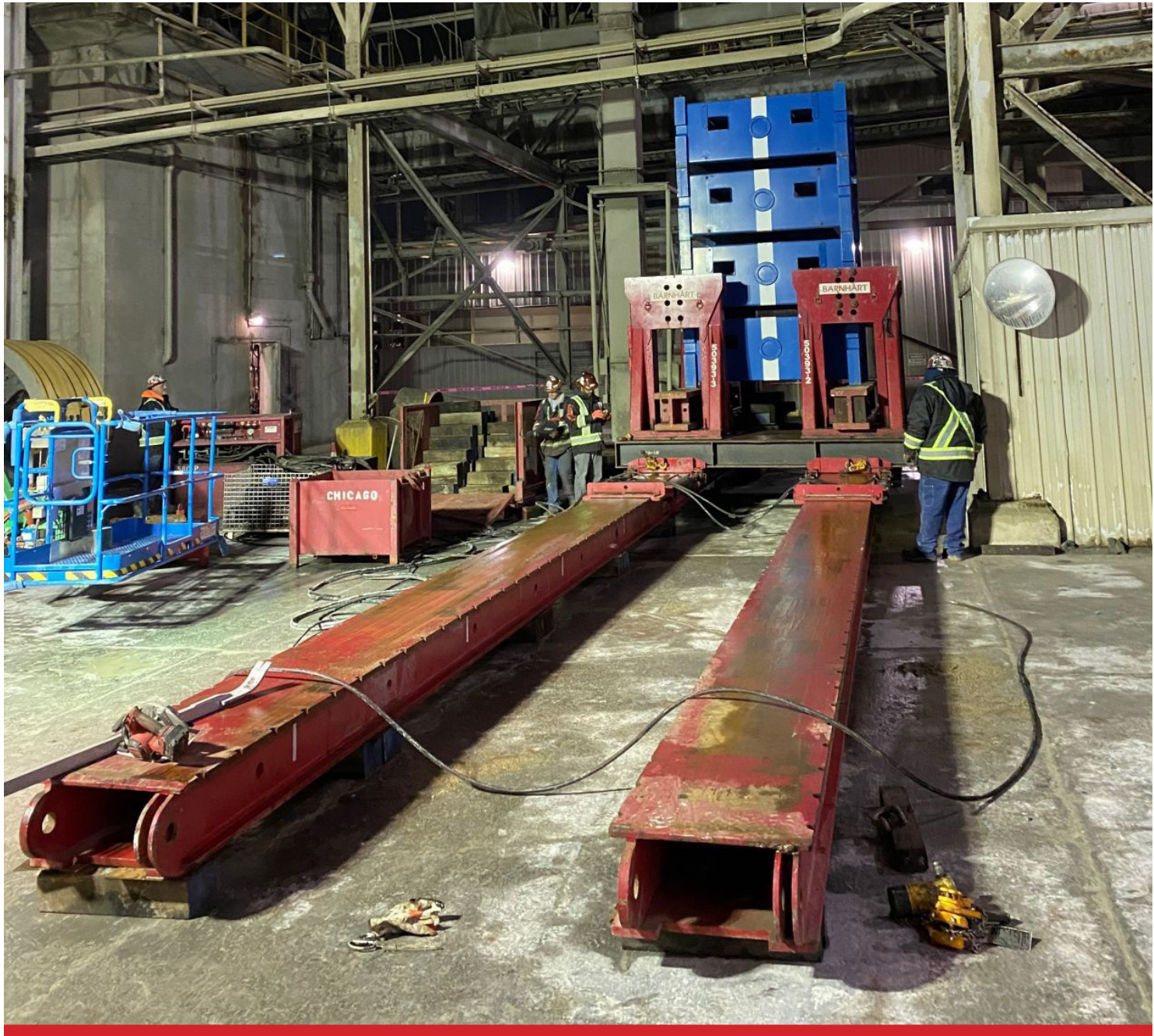
The crew installed 24" x 20' long slide beams and a 24" pusher gripper system that was used to build a shoring tower made of four BPU-750 barrels to slide under the cable tray.
