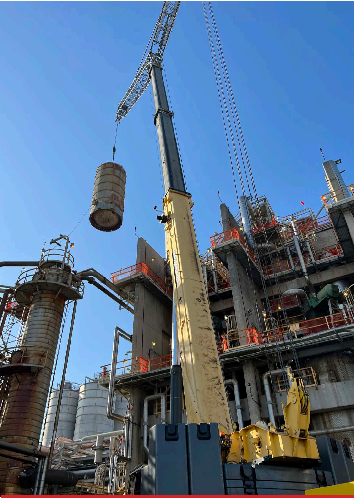
A 350-ton crane replaces a crystallizer vessel during an outage at a chemical plant.
