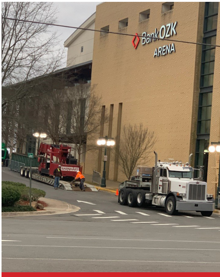
1 Barnhart was contacted to remove and replace a 22,000-pound escalator inside an arena in Hot Springs, Arkansas.
