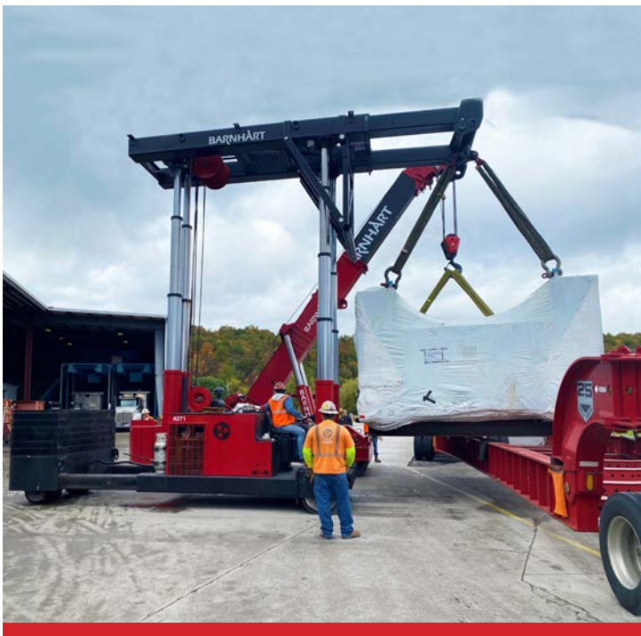
1 The Barnhart team helped with the installation of a 176,000-pound press at a manufacturing facility in Tennessee. The team first unloaded the press from a third-party trailer with a 75-ton MobiLift and 75-ton TriLifter.
