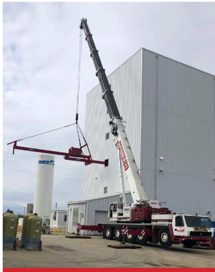
Barnhart utilizes the Movable Counterweight Cantilever System to rearrange components inside a facility in Decatur.
