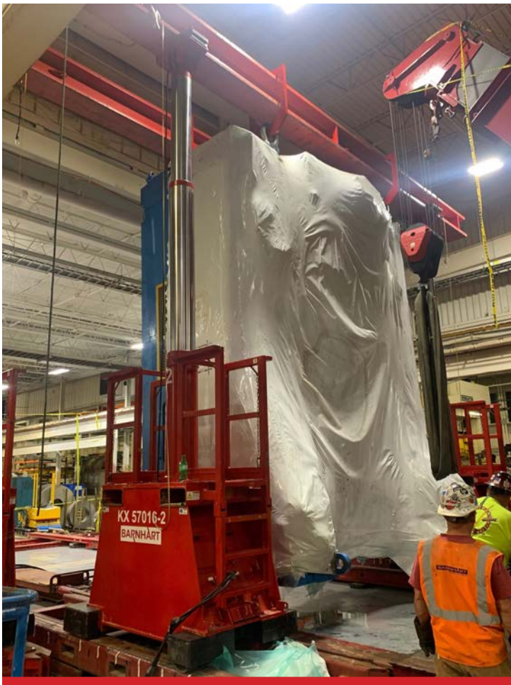
3 Using the MobiLift and 400-ton gantry system with track beams, the press was upended. Working conditions were very tight inside the plant for equipment setup and hauling.
