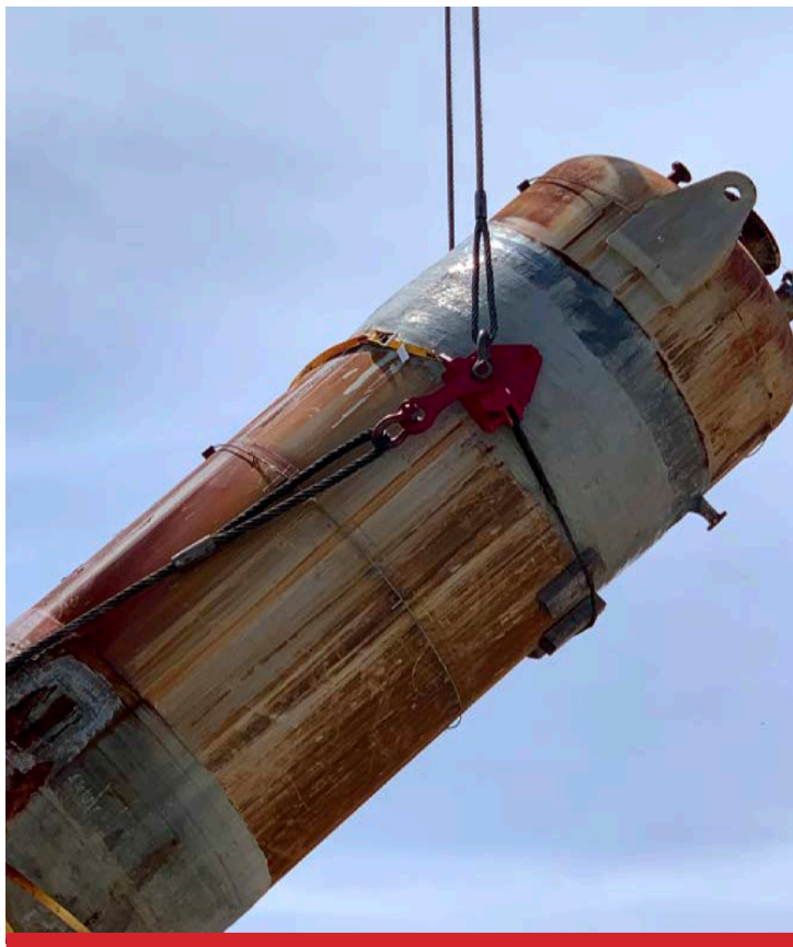
Temporary trunnions were used in the removal of this scrubber because its head lugs were corroded and unusable.
