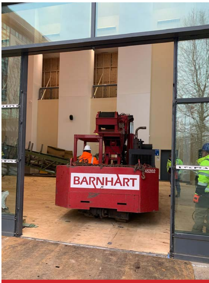
2 Barnhart proposed an option for removing and replacing the escalator using a Mobilift and 18K Hyster forklift, versus using an engineered scaffolding option from a different vendor.
