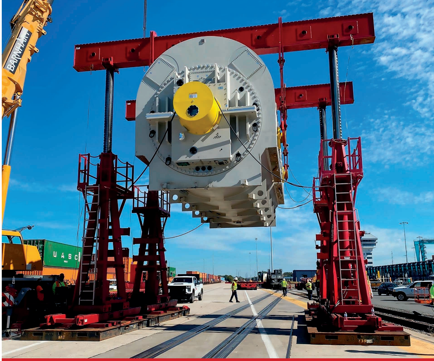
Lifting an 834,000-pound Siemens generator from a rail car using 500-ton one-shot gantries at the Norfolk International Terminal.
